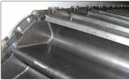
bucket conveyor for ash transportation
